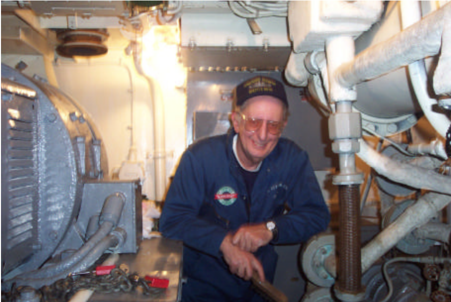
Cliff Nutter in the pump room
